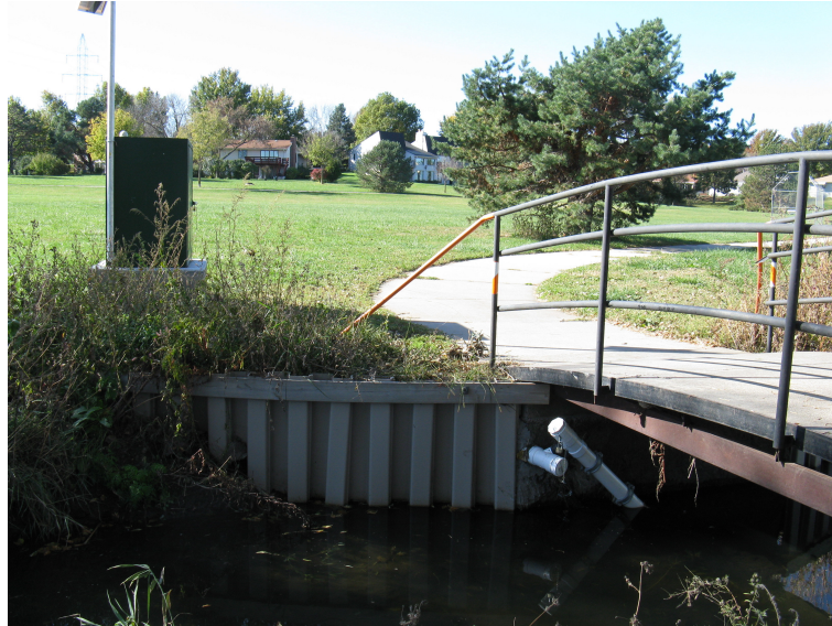
Figure 3.3: Probe Installation. The data probes are contained inside the white PVC pipe seen underneath the bridge here.
